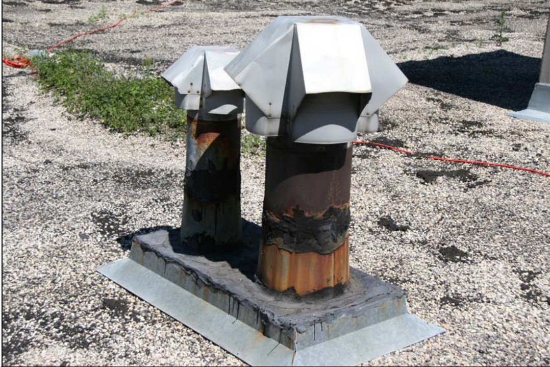
Photo # 7 This photo shows two existing old chimneys. No proper flashing or storm collars have ever been in place.
