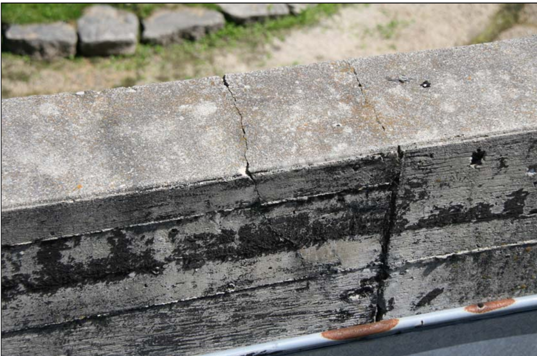
Photo # 14 This photo shows a fracture in the concrete parapet. The new roof should have the membrane carried up and over the parapet and a metal flashing installed.
