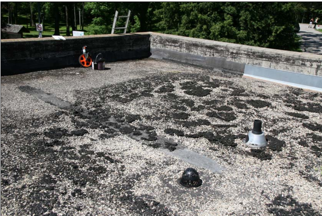
Photo # 10 This photo shows a location of the single roof drain. The roof drain is no where the middle of the roof and proper drainage does not occur.
