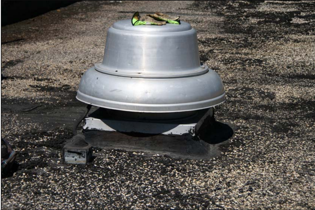
Photo # 9 This photo shows another fan unit with a proper pitch box in place.
