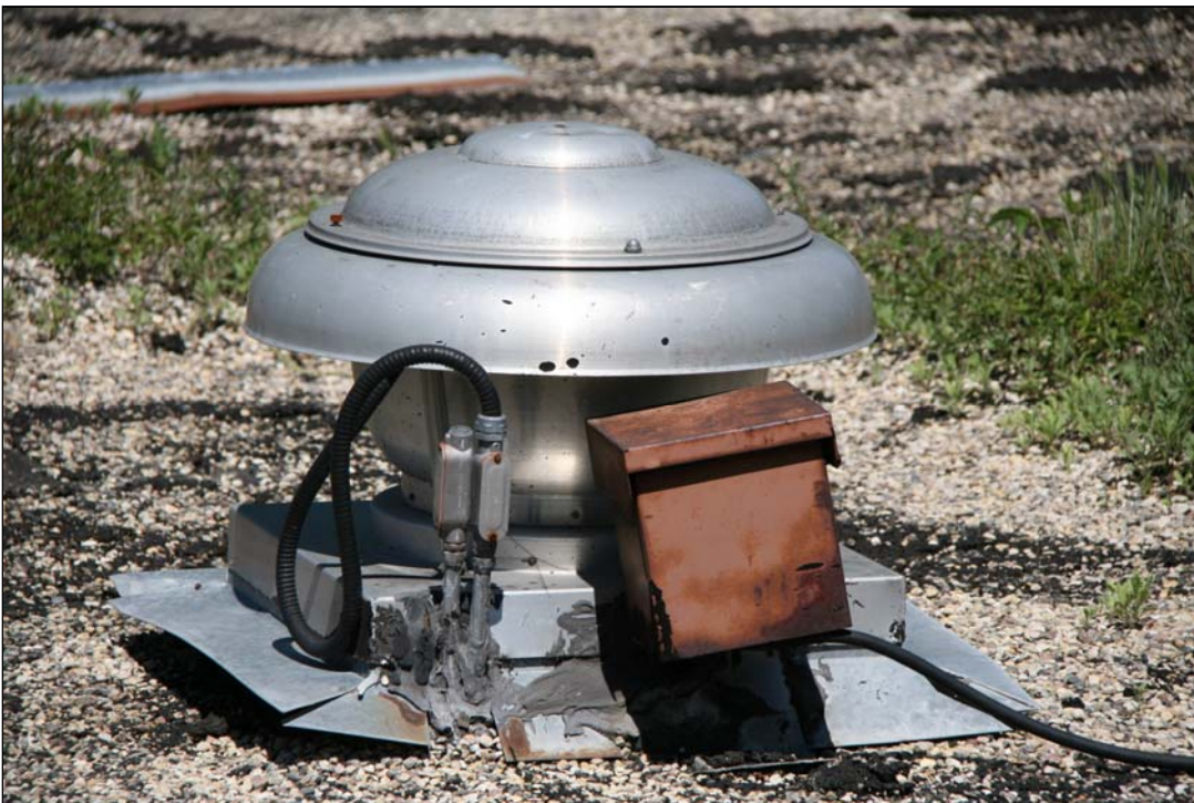
Photo # 8 This photo shows one of the fan units. Notice the conduits come up right against the unit and merely sealed with mastic. They should always penetrate the roof a minimum of 12" away so a proper pitch box can be installed.
