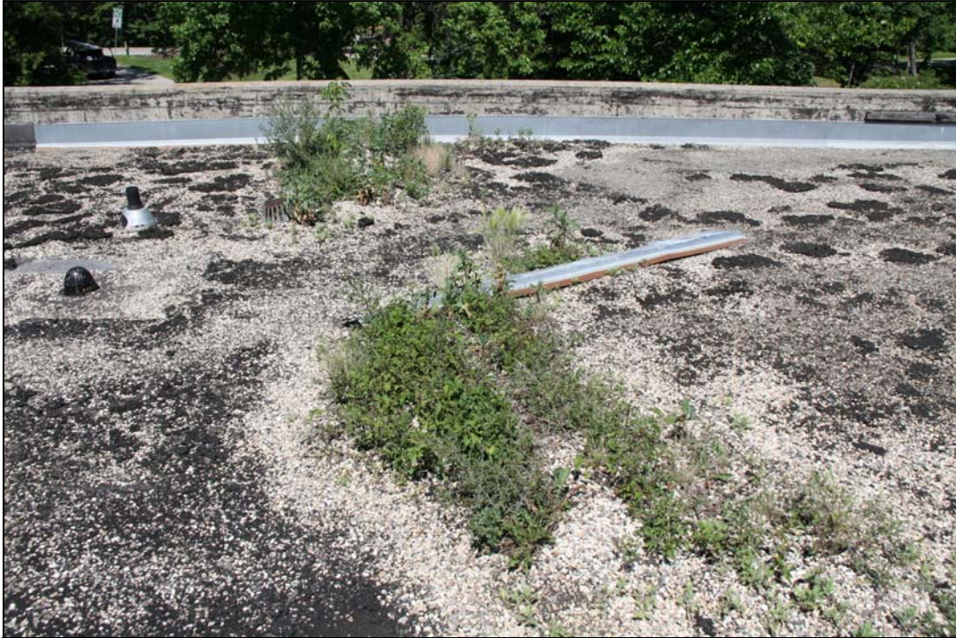
Photo # 11 This photo shows some of the plant growth on the roof.
