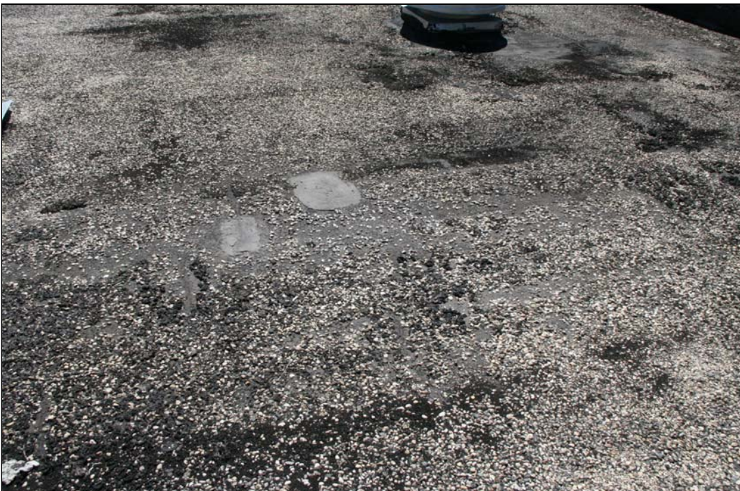
Photo # 12 This photo shows some of the numerous past repairs done on the roof.
